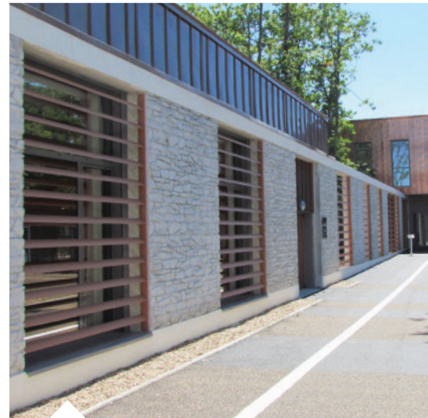
Middle School Montesquieu, ORLÉANS (45) Architect: Crea'ture architecte | Installation: Bernardi
