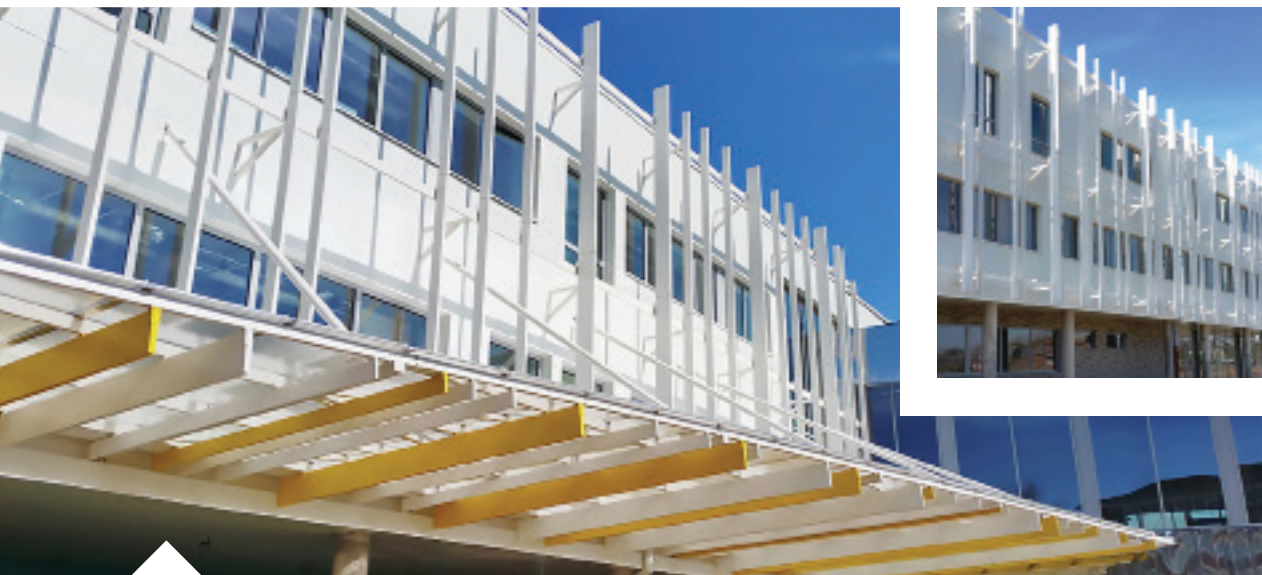
Middle School Eugène Thomas, LE QUESNOY (59) Architect: Scp Otton Sanchez Architectes | Installation: CMB Rousseau
