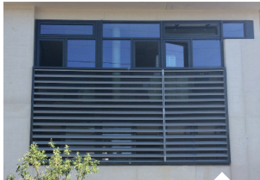
EDS, VILLENEUVE SAINT GEORGES (94) Architect: Jorge Magalhaes Architecte | Installation: CMH
